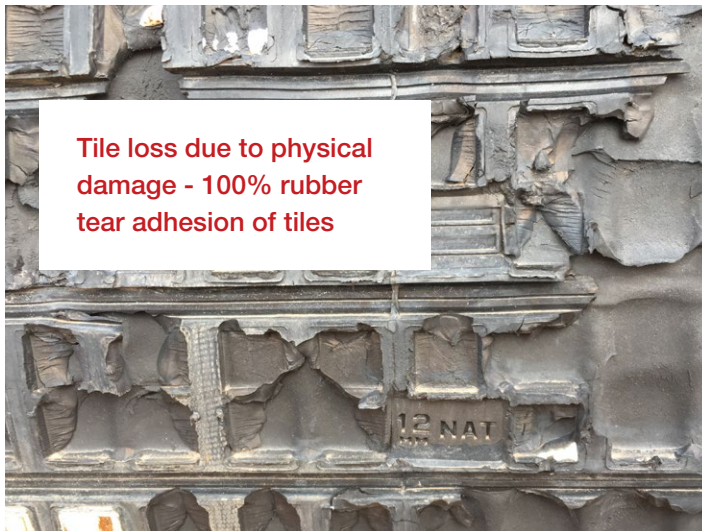
Photo#5 Tile loss due to physical damage.
