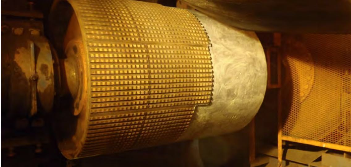
Image#1 - Lagging debonding
