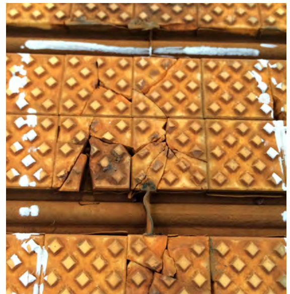
Image#3 - Tile cracking
