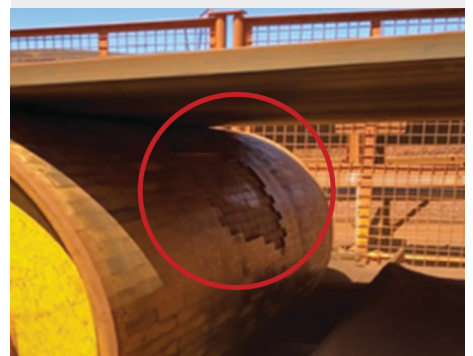
Tile debonding with existing lagging
