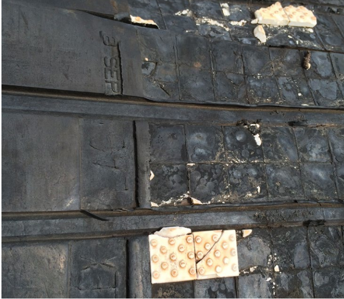
Ceramic tile loss due to debonding
