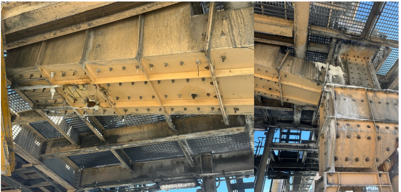
Leakage from studded wet plant causes corrosion, damage and risk
